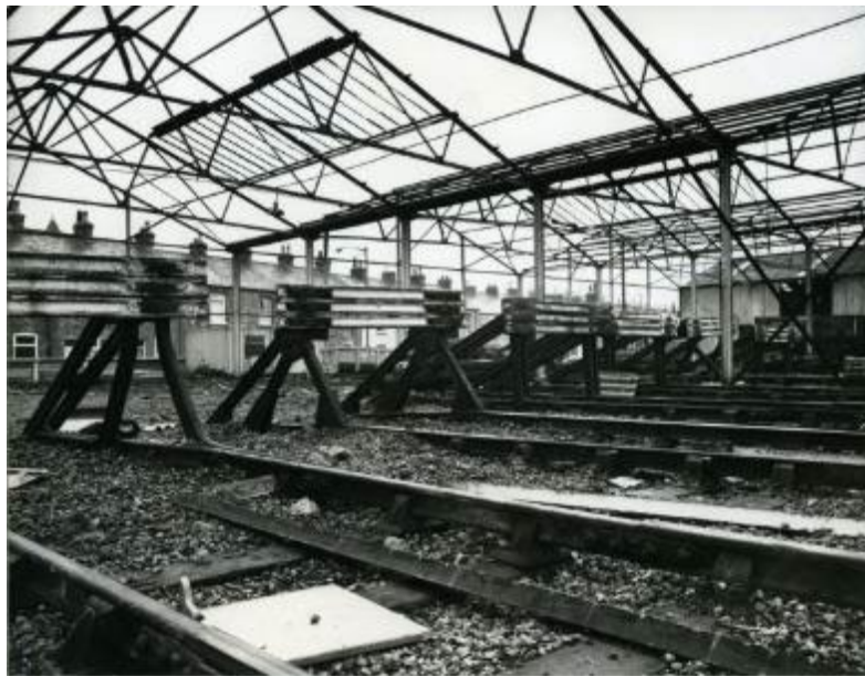
March 1980: A skeleton is all that remains of the 50-year-old carriage cleaning depot in Kingsland Terrace, which was being replaced by a new cleaning depot
